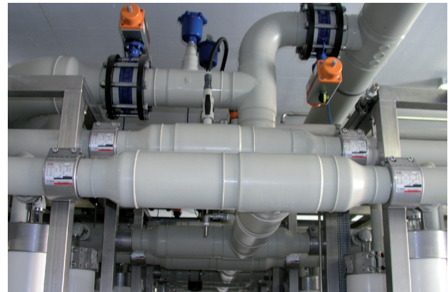
Water treatment application; connections between the racks
