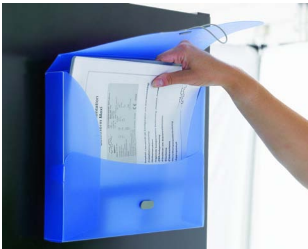
All documentation is placed in a binder behind electrical panel
